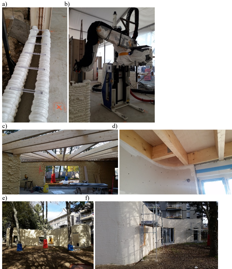
Fig. 7. The construction site of Yhnova™ – a) Deposition of the 6 first layers on the slab showing the reinforcement bars – b) Deposition of PU showing the AGV, the PAA and the protective tent – c) Timber frame for the roof – d) Inner curved plaster boards – e) Outer view of the walls – f) View of the wall covered with external coating.
