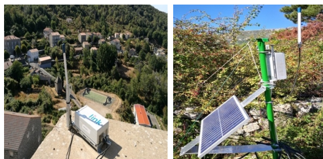
Figure 4. LoRa Antenna for the Smart Village on the church roof (left) and second rescue antenna with solar panel (right)
