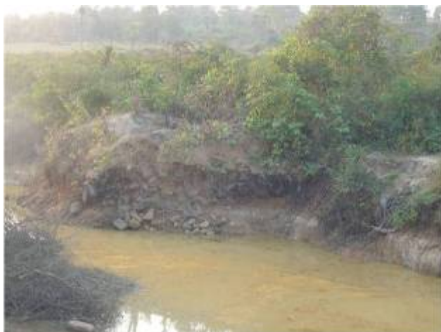
Figure 12. Massive masonry structure in the western face of the east bank of the West Baray (Fletcher).
