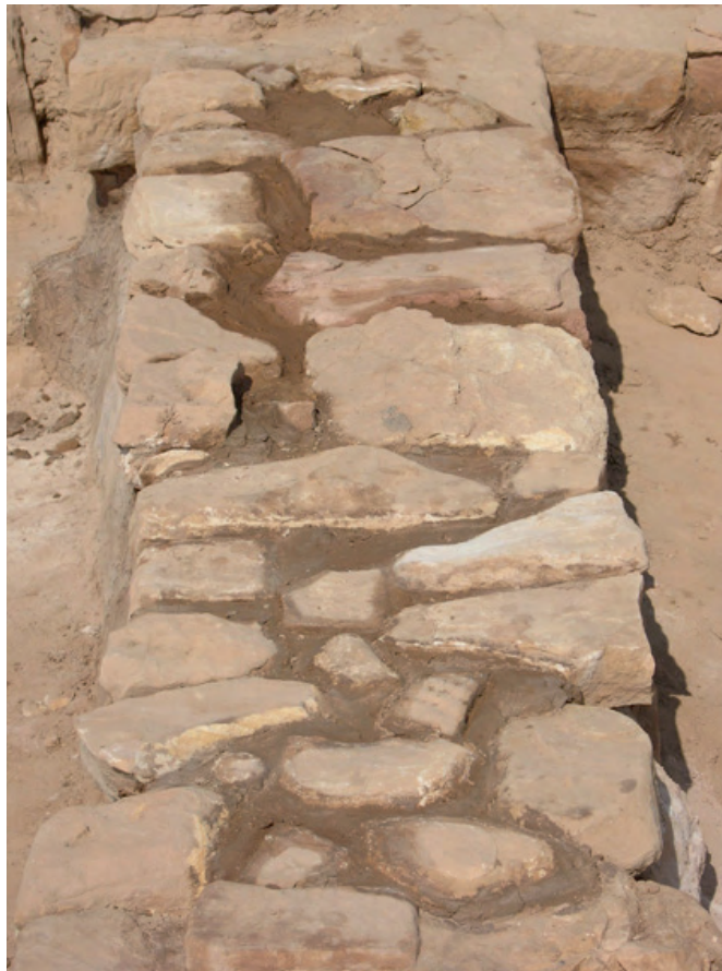
Fig. 27. The joints of the top of the wall have been filled with mortar. Some of the missing parts have been rebuilt with the same materials as those used in antiquity.
