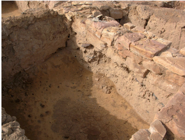
Fig. 32. Room 5, east wall, undermined wall.
