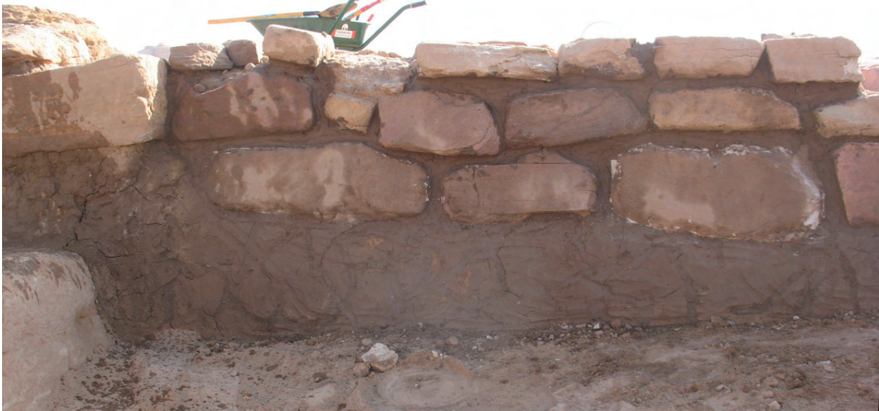
Fig. 26. The joints of the walls have been filled with mortar and the base, which is to be exposed, is reinforced by a bench made of small stones and mud.
