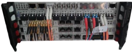
Figure 4: Example of VME rack used.
