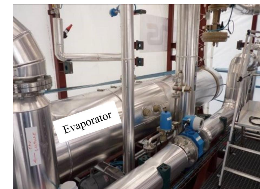
Flooded shell-and-tube evaporator
