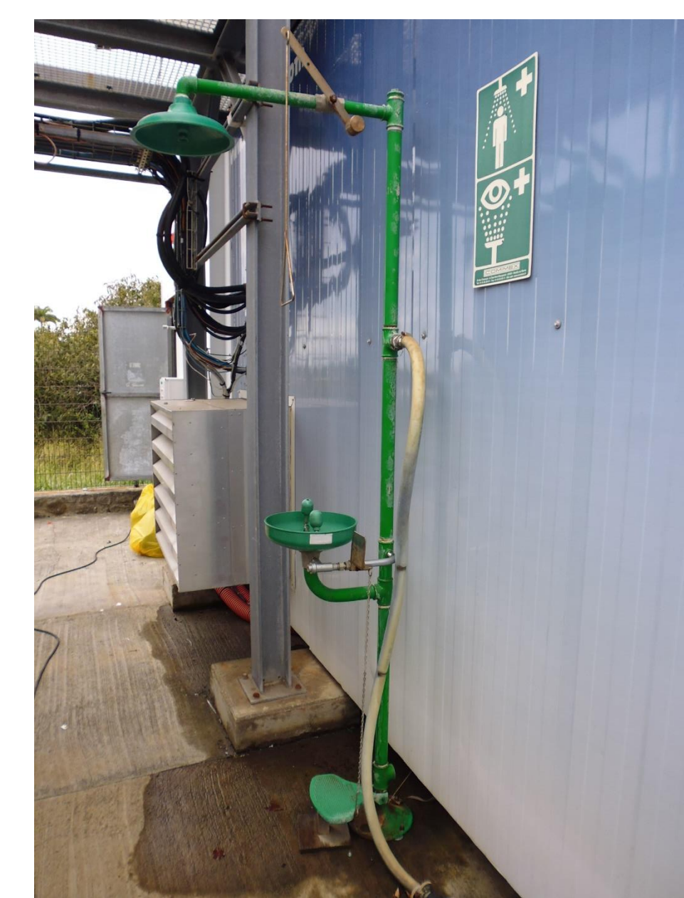
The security shower in case of contact with ammonia
