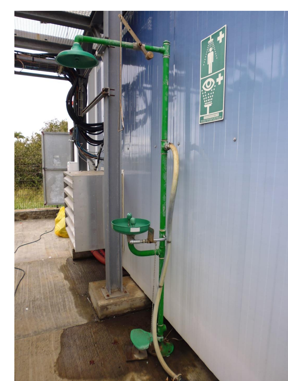
The security shower in case of contact with ammonia
