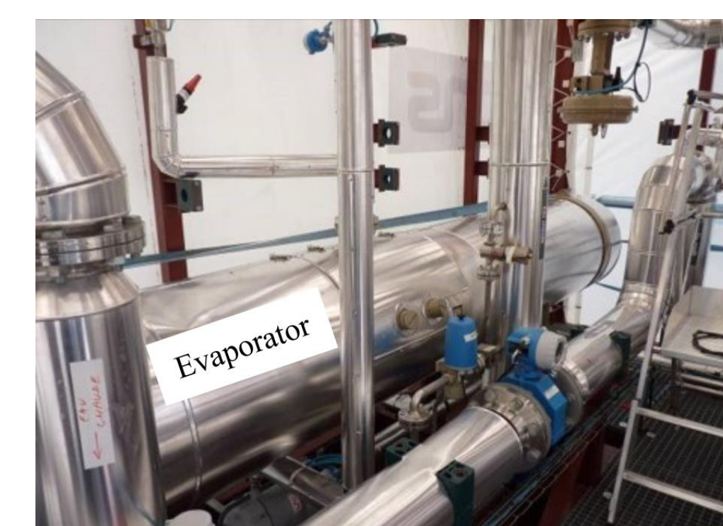
Flooded shell-and-tube evaporator
