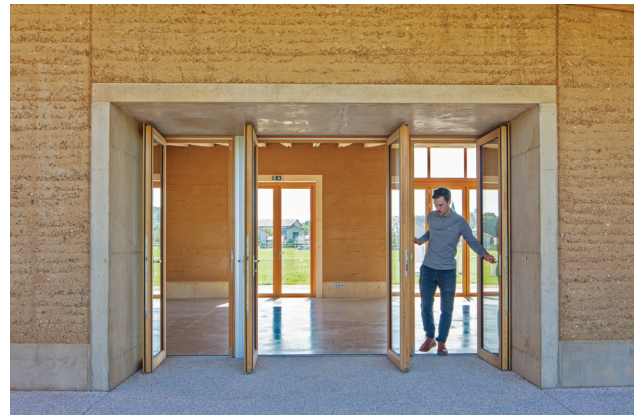
△ Figure 9. Concrete moment frame and chamfered control joints at west rammed-earth wall. (Credit: Eduard Hueber / archphoto)
