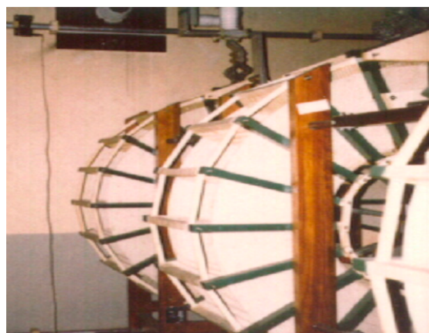
Figure 5. Three phase reactance in the power station “Folies”.
