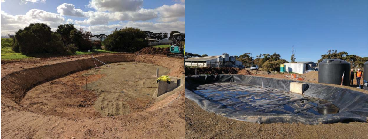
Plate 2 The outline of high rate algal pond with the completed dam wall and pond liner (June 2017).
