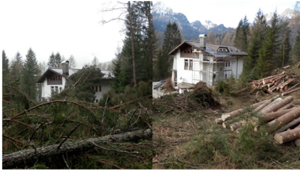
Figure 1 Left: Centre of Studies for the Alpine Environment (Belluno, Dolomites, Italy) on October 30, 2018, on the day after the event. Notice fallen trees on the roof of the building and part of the damages done in its vicinity. Right: Same position two months later (January 4, 2019), with the first restoration works (Photographs: Roberto Menardi).
