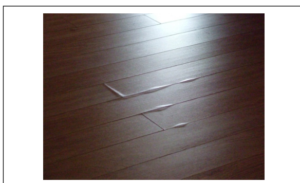
Fig. 1 : Example application of MDF: flooring, having suffered water damage
