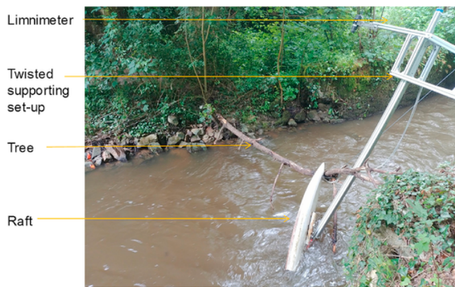
Fig. 12. View from the bank before reparation work.
