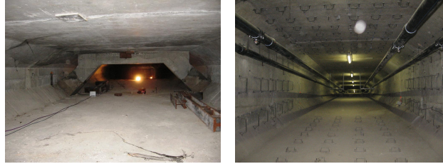
(a) View inside box before strengthening. (b) View after strengthening external with prestressing cables installed in the bridge deck.
