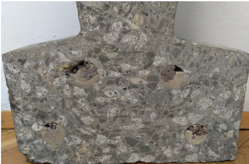
Fig. 6 Unproperly filled lower cable ducts on cut out cross-section of the tested beam.
