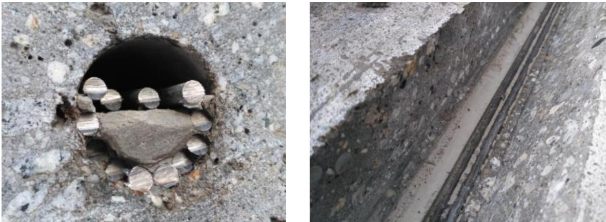
Fig. 5 Front view of prestressing cable (left) and opened cable duct view (right).
