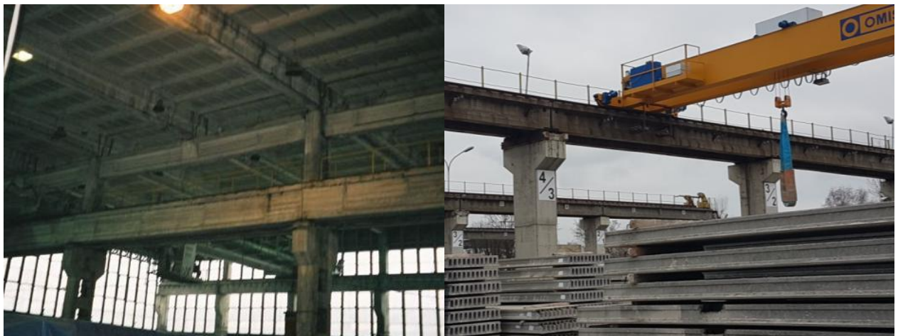
Fig. 1 Post-tensioned beam track for the overhead cranes inside the industrial plant (left) and external post-tensioned beam track for the overhead cranes (right).
