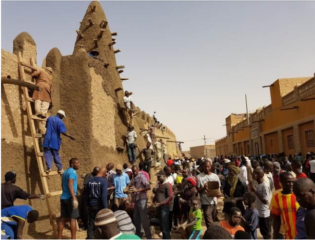
Figure 8. Traditional plastering of Djingarey-ber mosque by the masons and the community of Timbuktu on February 19, 2017. © UNESCO - Bagayoko M.
