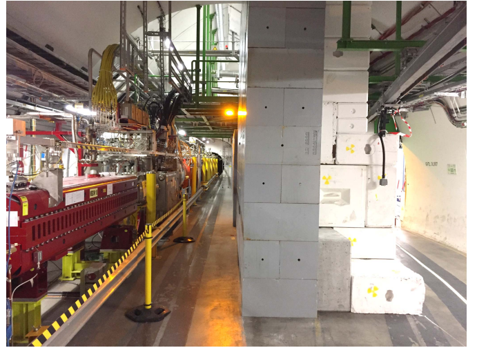
Fig. 4. Photograph of UJ14. The tunnel to the left just before the ATLAS experiment and the shielded alcove to the right.
