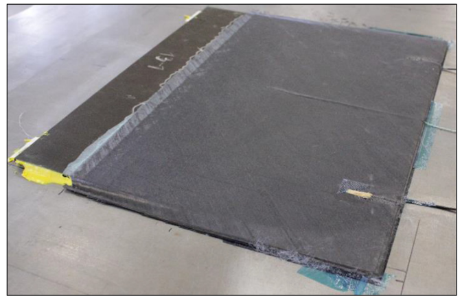
Fig. 14. View of finished repair on “Plate 13” after curing (overlap length of 13 mm).
