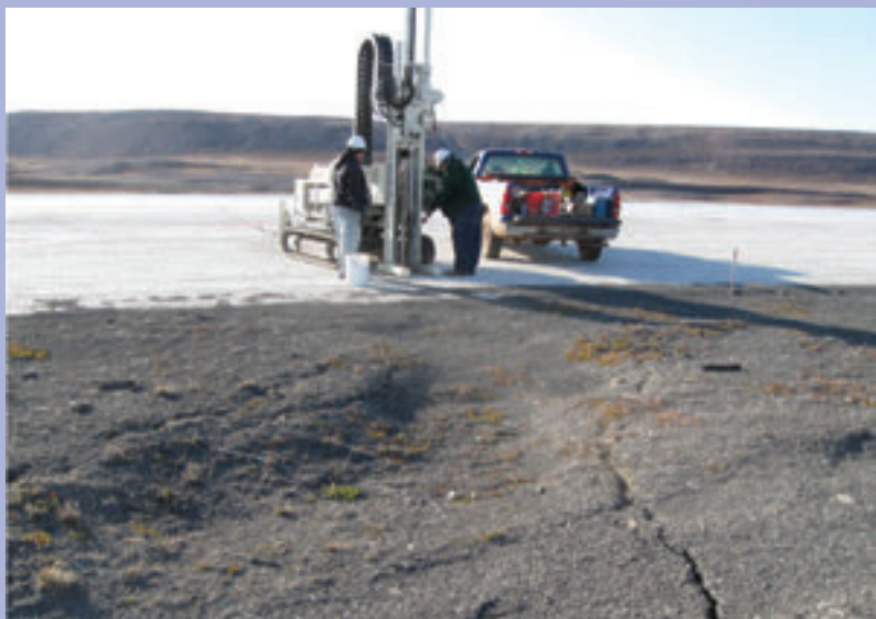
FIG. SB5.4. Thaw settlement (~0.65 m) associated with an airfield in Greenland. Thawing of ice-rich, weathered bedrock at approximately 2 m below the surface is causing severe settlement, resulting in the need for significant maintenance measures to continue operations. Photograph by Kevin Bjella.
