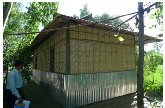
Wall with three parts: iron sheets in the bottom part (more resistant to moisture); thick bamboo panels to ensure privacy in the middle portion and thin ones in the upper part to allow ventilation (Rangpur). © A. Caïmi
