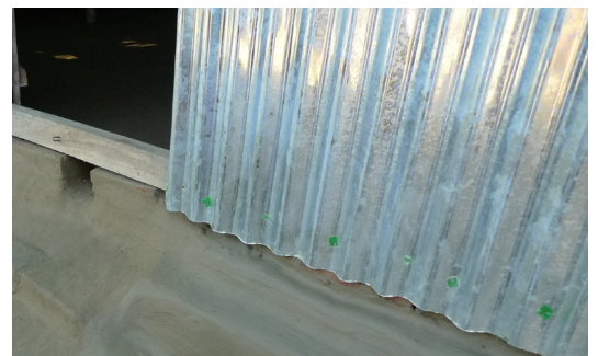
Plastic bottle pieces as washers between the nails and the CGI sheets to avoid the deterioration of iron sheets by the nails during strong vibrations under wind pressure (Dinajpur). © A. Caïmi
