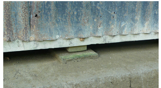
Concrete plots ( katla ) to keep moisture from rising into the wooden structure and gap between walls and soil in Kuakata (Barishal). © O. Moles
