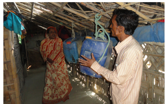
In case of light roofs in flood-prone areas, empty jerrycans are sometimes fastened under the roof structure. During high floods, the roof is detached from the main structure (or loosely connected to it) and the jerrycans work as floats avoiding a complete sinking of the roof (not a very common practice). © O. Moles
