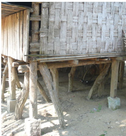
Wooden posts often rely on one or more implanted waterproof elements (Bandarban, Chittagong). © O. Moles
