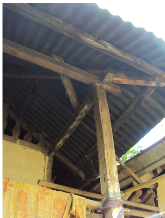
Corner bracing keeping the structure from bending under lateral loads due to earthquakes or strong winds (Sylhet). © A. Caïmi
