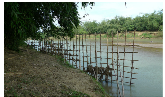
Bamboo grids built on river banks exposed to erosion, working as wave breaker and helping control earth erosion during floods (Mymensingh). © A. Caïmi
