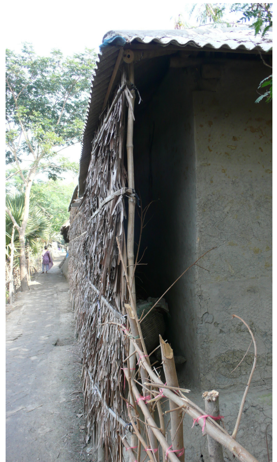
Wall protection according to orientation in Ashashuni, Khulna. © O. Moles
