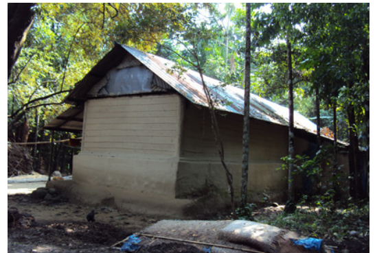
Lower parts of the walls are built with earth (cob), burnt bricks or cement blocks, and upper parts with reed mats, bamboo mats or iron panels (Sylhet). © O. Moles
