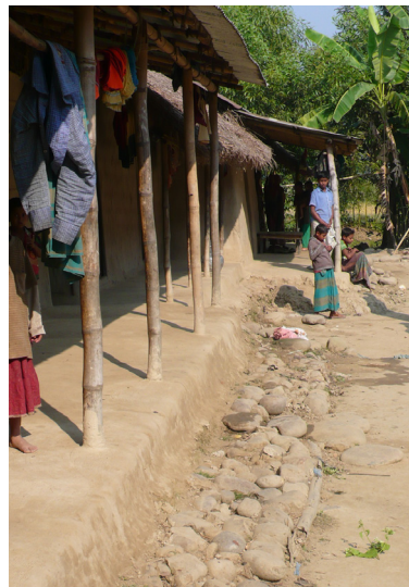
Plinth protection with stones, also used to prevent erosion due to water falling from the roof (Sylhet). ©O. Moles
