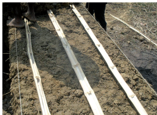
Bamboos are sometimes embedded into cob walls. They improve the behaviour of the wall under horizontal seismic stresses (Rajshahi). © sos-arsenic.net
