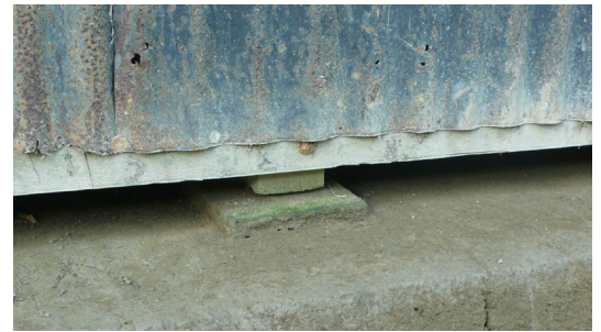
Concrete plots ( katla ) to keep moisture from rising into the wooden structure and gap between walls and soil in Kuakata (Barishal).
