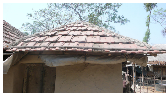
Tiled roof fastening against strong winds effects in Khulna division. © O. Moles
