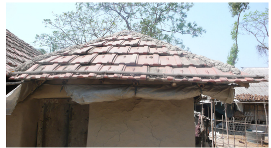
Tiled roof fastening against strong winds effects in Khulna division. © O. Moles
