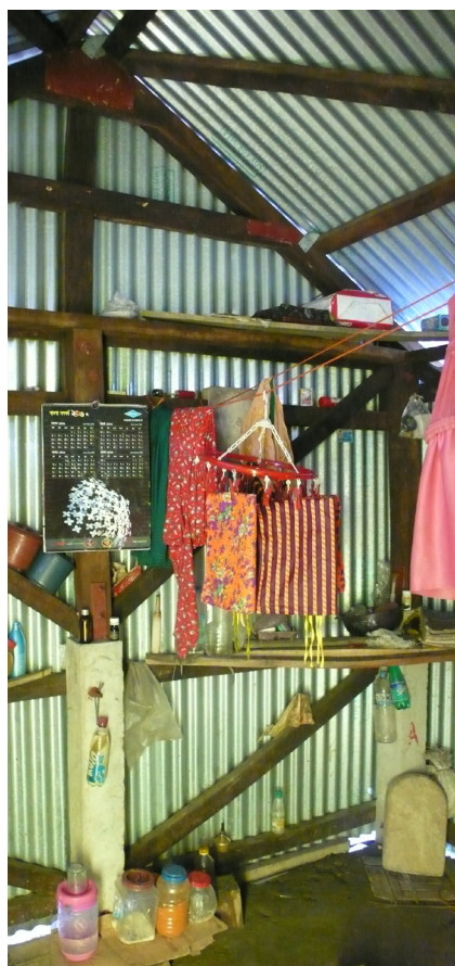
Wooden bracings and katla (concrete plots) in Barishal. Project by DFID and BRAC University. © O. Moles
