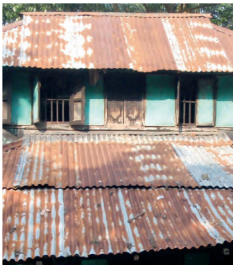
Corroded CGI roofing in coastal area (Kalapata) ©IFRC-SRU
