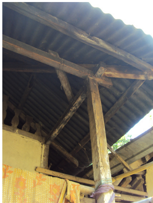
Corner bracing keeping the structure from bending under lateral loads due to earthquakes or strong winds (Sylhet). © A. Caimi
