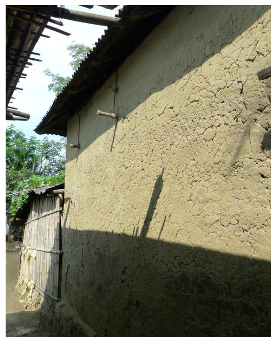
The roof is tied to bamboo pieces embedded through the walls (Mymensingh). © A. Caïmi
