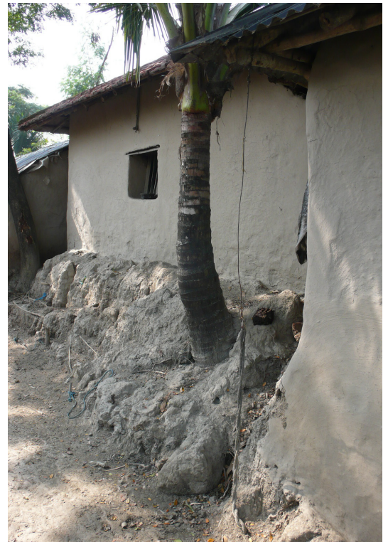
Roof anchored to roots in Khulna. © O. Moles
