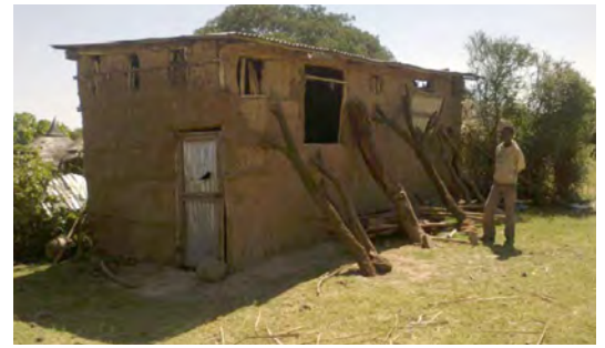
Termite infested house supported by poles. © D. Debelo & E. Degaga
