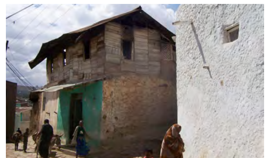
Heavy ground floor and light upper floor in Harar. The upper parts of the walls have a decreased thickness and/or are built with materials lighter and more flexible than those used for the lower parts. CC- Beth
