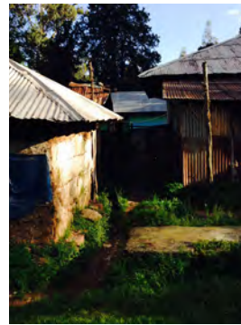
Hipped roofs with better resistance to strong winds in the Ethiopian highlands. CC- Beth
