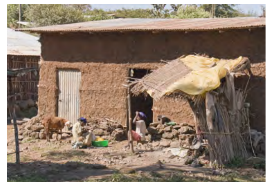
Stone masonry wall built to protect the lower part of the chikka walls in Bahir Dar. (Amhara). CC- A. Davey
