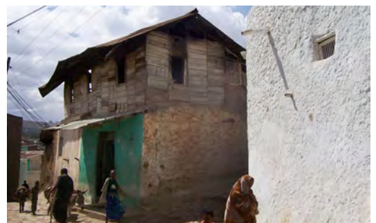
Heavy ground floor and light upper floor in Harar. The upper parts of the walls have a decreased thickness and/or are built with materials lighter and more flexible than those used for the lower parts. CC- Beth
