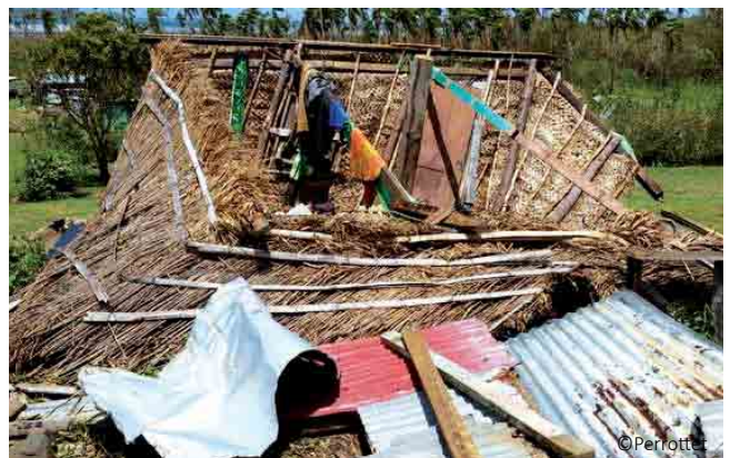
Construction with mixed materials: even if heavily affected, its lightweight limits risks of serious injury.
