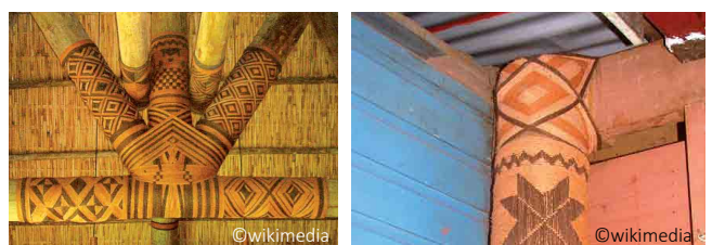
Coconut fibre tying for roof trusses (left) and corner post-ring beam (right).
