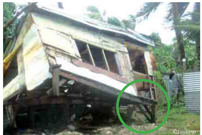
Even if other vulnerabilities have led to serious damages, corner bracing under the platform is an important feature to improve the house stability.
