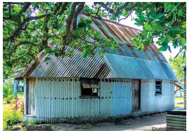
Bure built using CI sheets as evolution of the traditional building practices: round shape for improved aerodynamism.
