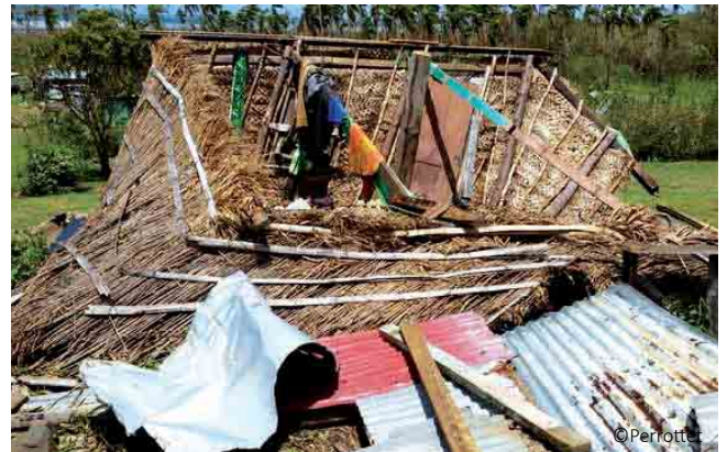
Construction with mixed materials: even if heavily affected, its lightweight limits risks of serious injury.
