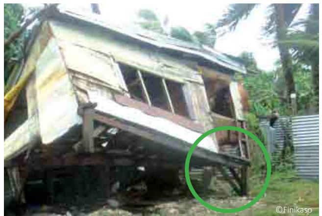
Even if other vulnerabilities have led to serious damages, corner bracing under the platform is an important feature to improve the house stability.
