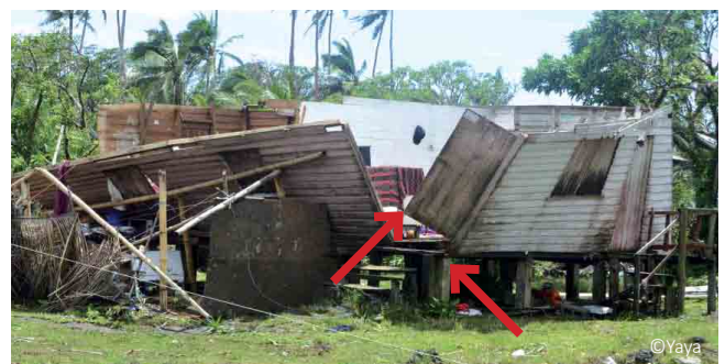
“Box explosion” under wind pressure due to weak connection between walls. Lack of anchoring between the corner posts and the concrete foundations.
