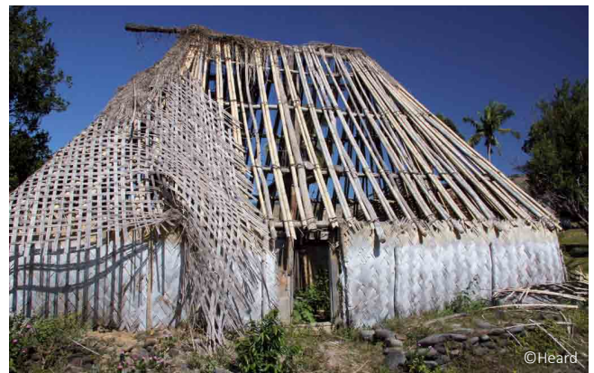
House damaged by a cyclone: a large quantity of materials can be reused for repair the existing house or to built a new one.
