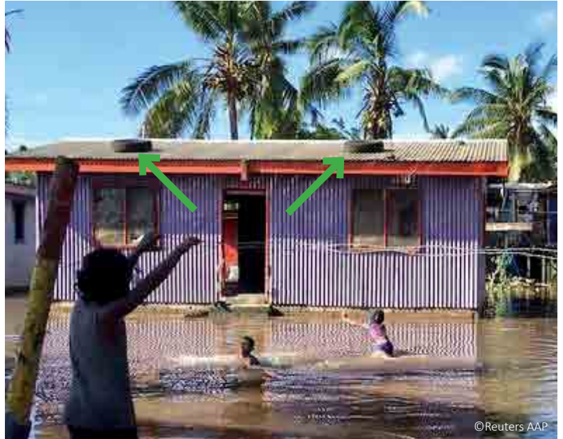
Tyres placed on CI sheet roof to reduce vulnerability to wind.
