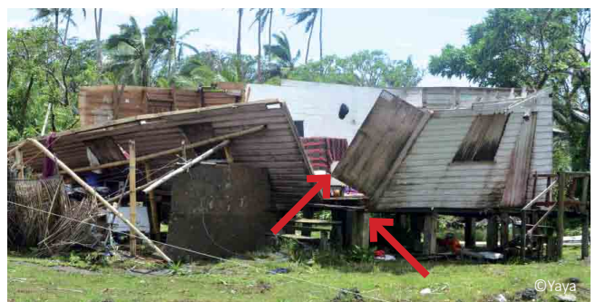
“Box explosion” under wind pressure due to weak connection between walls. Lack of anchoring between the corner posts and the concrete foundations.
