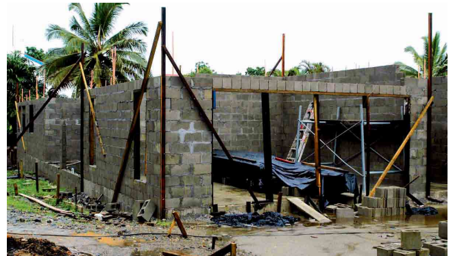
Poor quality cement block masonry house with steel rods.
