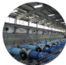
LADWP Filtration Plant
