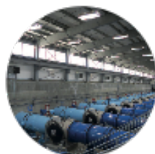
LADWP Filtration Plant
