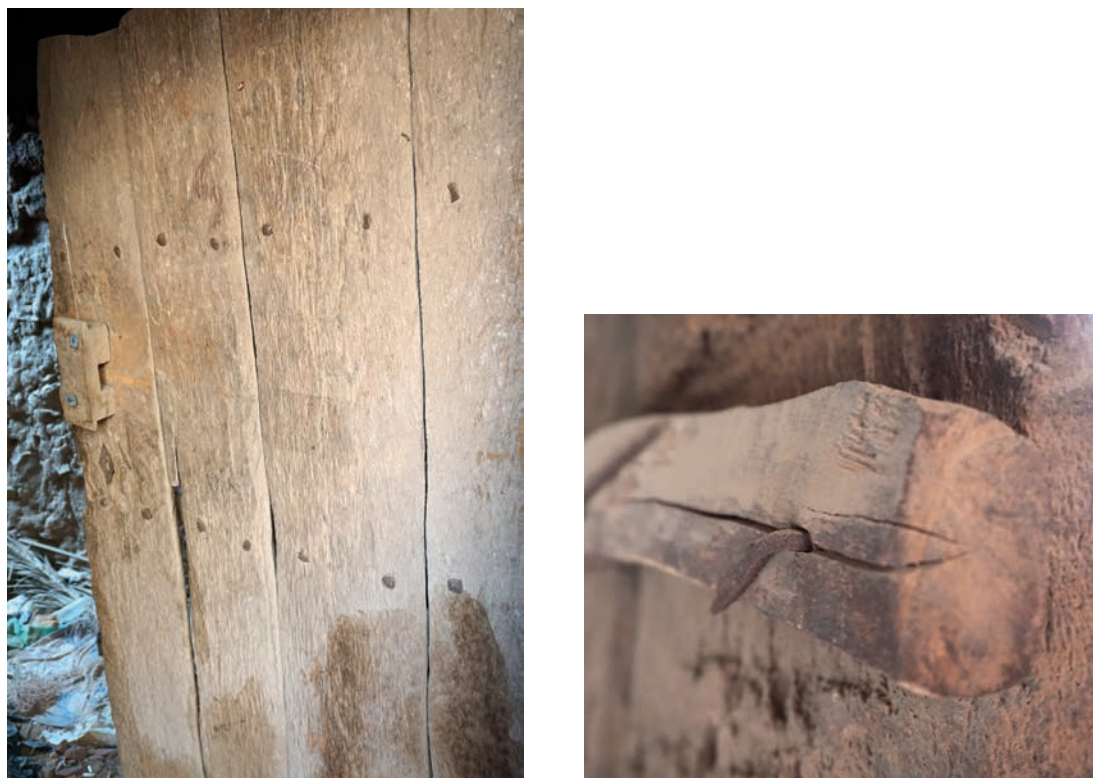
Fig. 2. Modern door in the old city of al-'Ulā, made of several sections of date palm trunk (a) joined together with a transversal beam (Tamarix) and nails (b).
