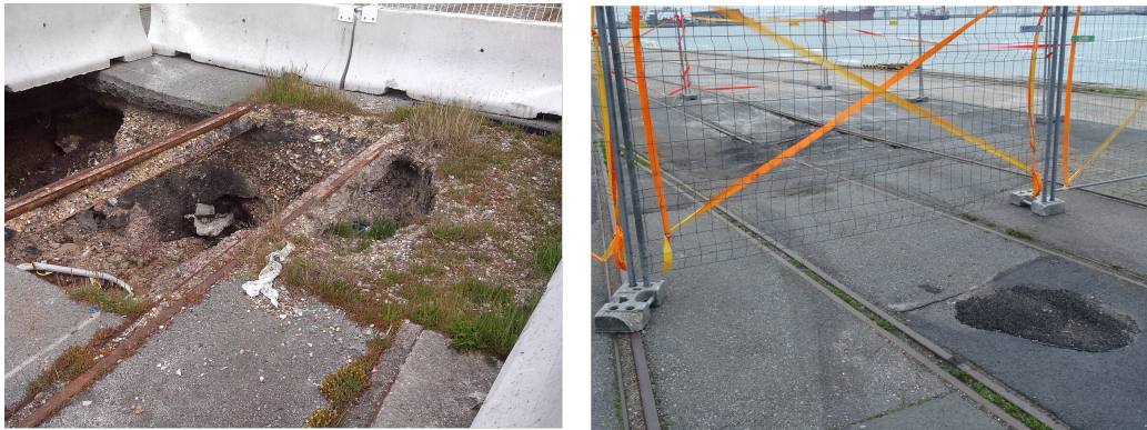
Figure 2: Photo of typical collapse and deformation observed these last years on the Joannes Couvert quay.
