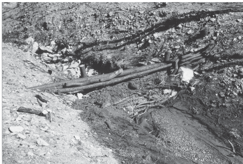
Figure 2. Log debris dam (LDD) showing trapped sediment and debris upstream of dam.
