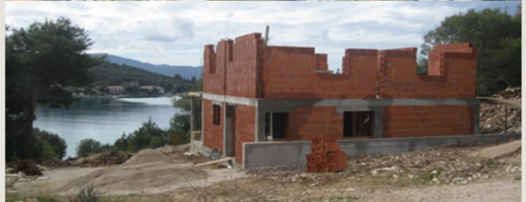
Due to weak government enforcement tourism development is accompanied by significant construction activities (AgroParisTech, 2017:111)
