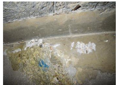
Fig. 10. Example of cracks located in the patch repair at diaphragm/shell junction.
