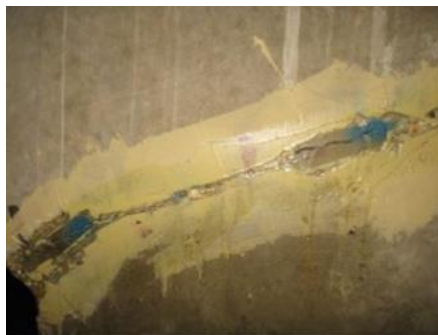
Fig. 9. Example of an injected crack detected in the diaphragms of the vault.
