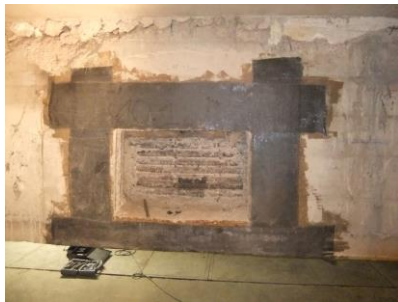
Fig. 11. Opening of a window in the tie after a local strengthening by CFRP.
