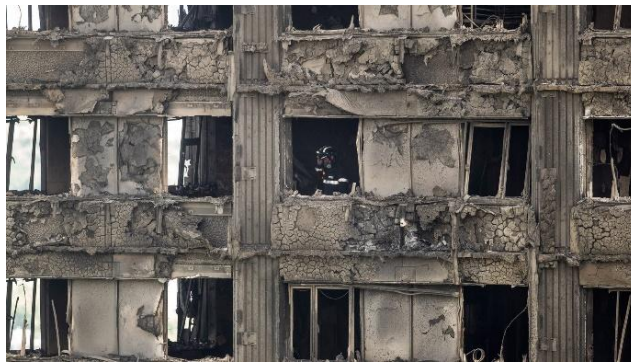
Fig 1. Facade of the Grenfell tower in the aftermath of the fire.
