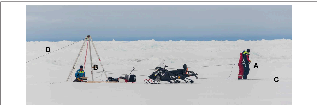
FIGURE 6 | Overview of the recovery procedure. Two persons (A) pull up the load with the 2:1 pulley system. The loop pulley rope is fixed in the ground (C) and diverted in the multiplier block (B). Note the guy rope (D) that is necessary to keep the tripod from tipping over. Picture was taken during the training session, where a bigger tripod was used. No Skidoo was available during the actual recovery.
