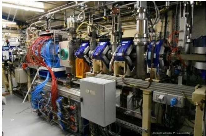
FIGURE 2. Photo of the SP1 Charge Breeder installed the middle of the LEBT.
