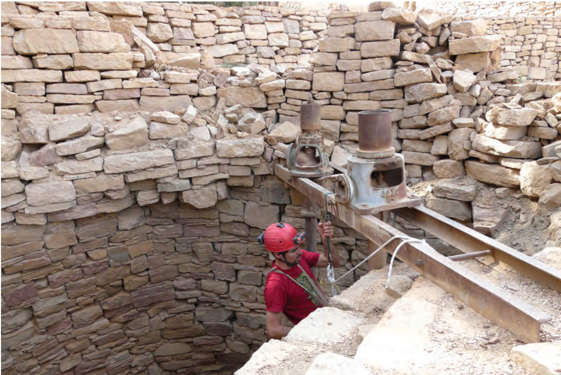
Fig. 10. Pumps with back screws are set up at the top of wells (here PU160)
