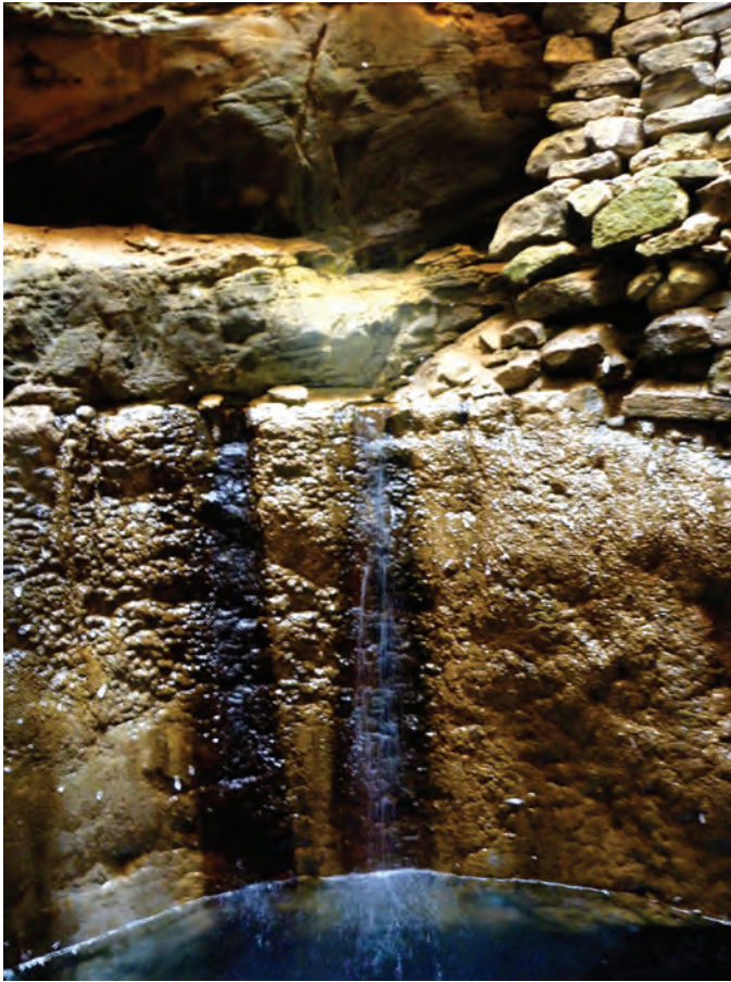
Fig. 18. Important infiltrations, visible in several wells, mainly at the joints rocky strata
