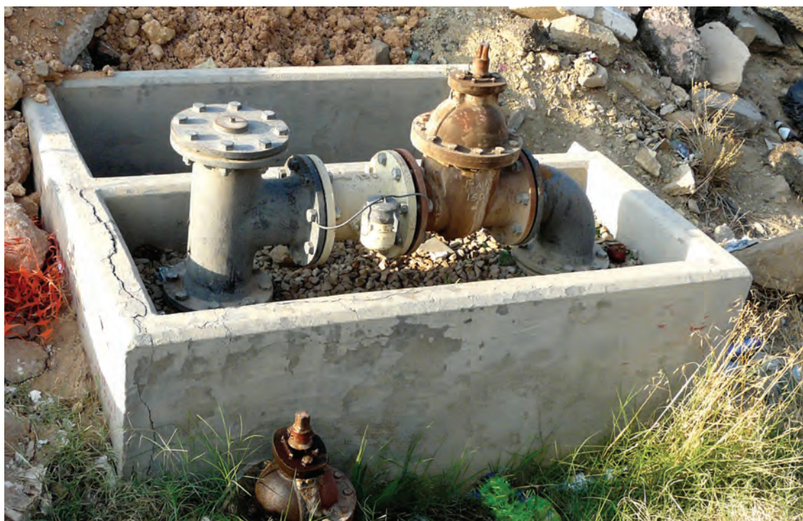
Fig. 12. New system fed by big pumping stations
