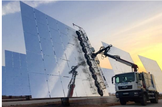
Figure 4: High pressure cleaner vehicle with cleaning brushes
