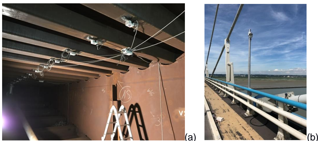
Figure 6 – SiWIM in the Normandy bridge: (a) extensometers under the longitudinal stiffeners in the box, (b) camera on the bridge deck
