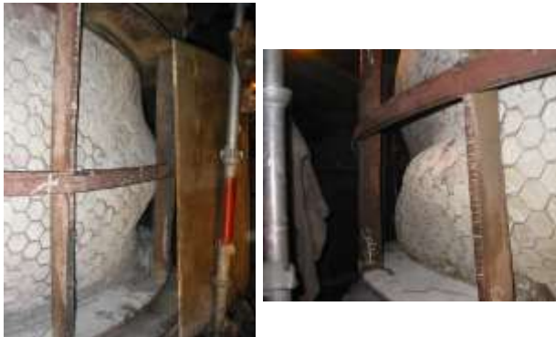
Figure 1. Typical deformation patterns at the riser bottom. Source: The authors.
