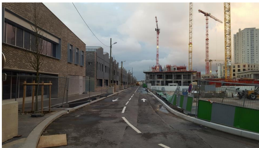
Figure I.11: Chapelle International Sogaris logistics hotel building site, February 2018 Source: photo Nicolas Lazarevic
