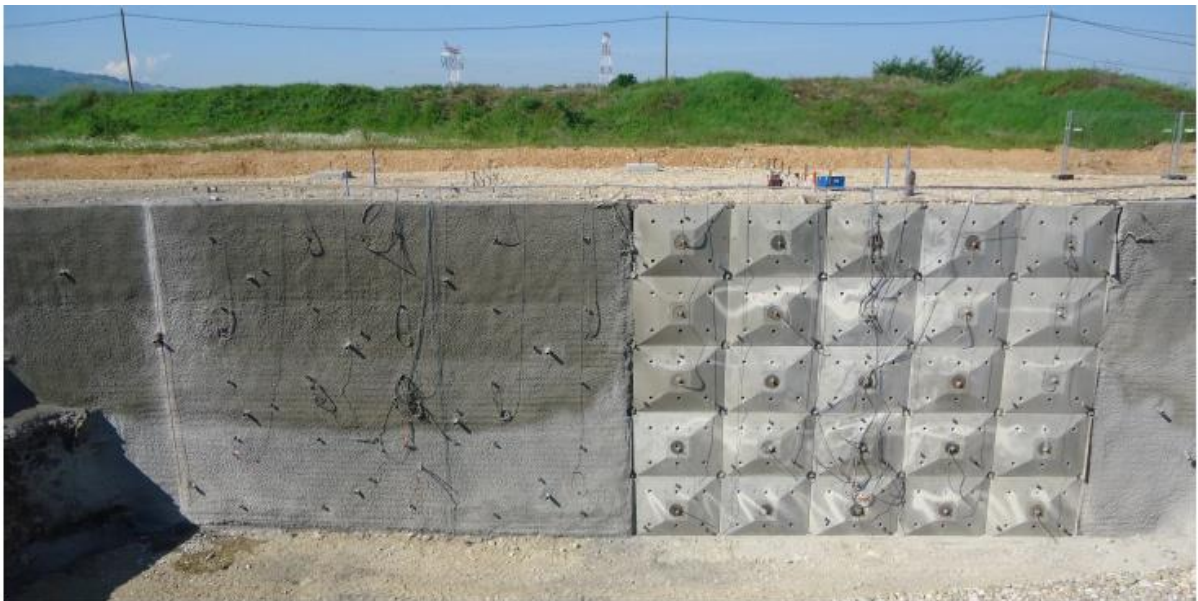
Figure 9. In situ full-scale soil nailed walls built in Bevenais, France (left side, shotcrete facing – right side, precast panels)
