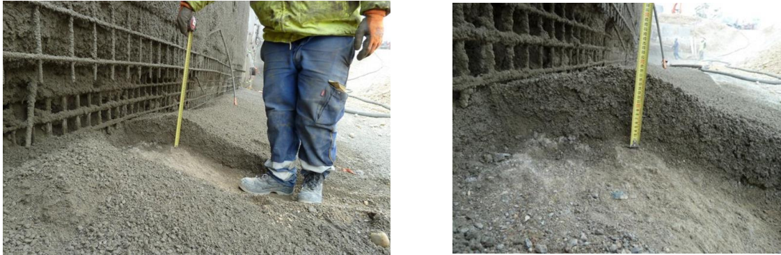
Figure 11. Wasted concrete due to rebound during shotcrete application
