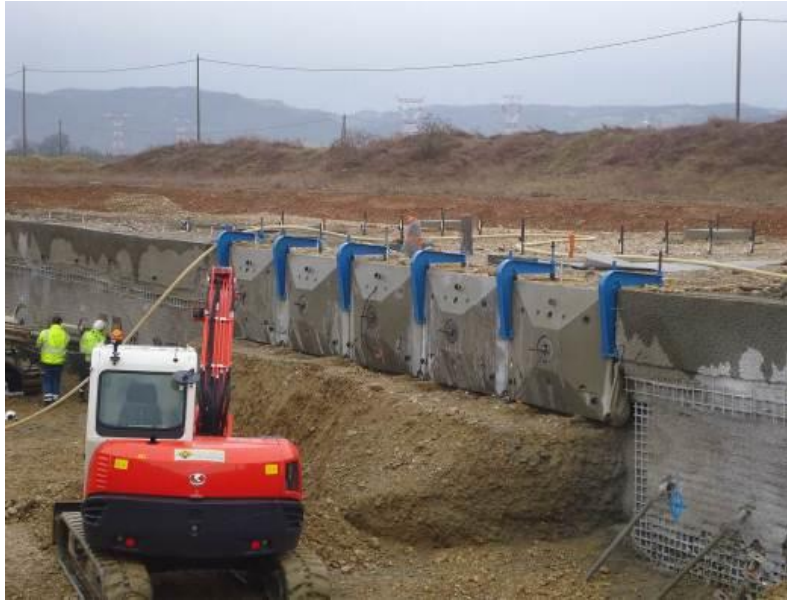
Figure 13. Temporary suspension brackets to avoid vertical sliding of the first panel row
