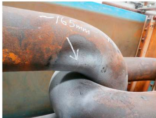
Fig. 15. Fatigue crack at the Kt position.
