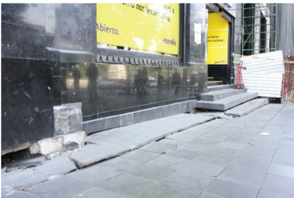
Figure 9: Evidence of soil-structure interaction in Mexico City (Photo courtesy of S. Brûlé and A.F.P.S. [69]).
