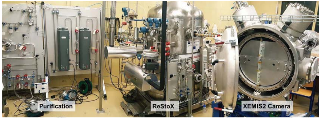
Fig. 2. Overview of the XEMIS2 cryogenics facility
