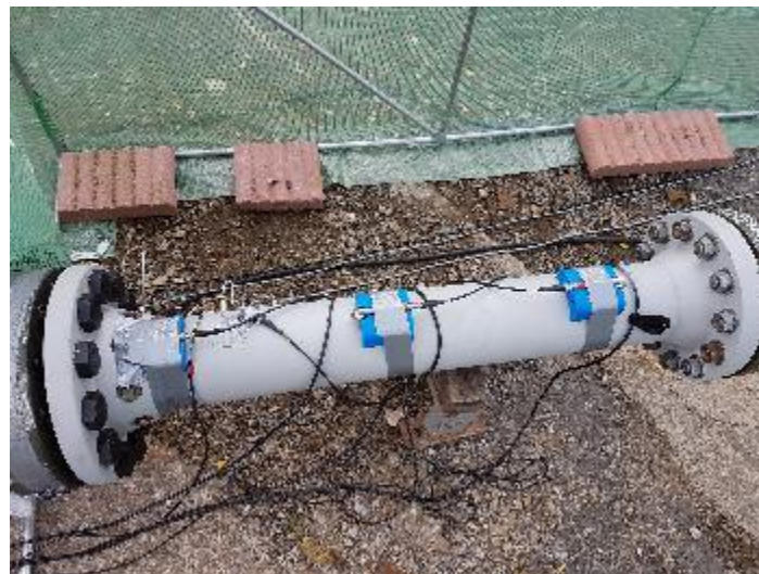
Figure 3 – Measuring spool equipped with its probes
