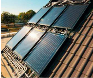
Fig.4 : Photos of the PV-T modules installed on the roof of BESTLAB
